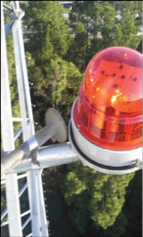
New LED obstruction lighting on microwave towers.
