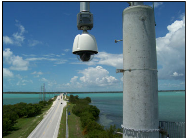
Closed-circuit television camera supports traffic management in Monroe County.
