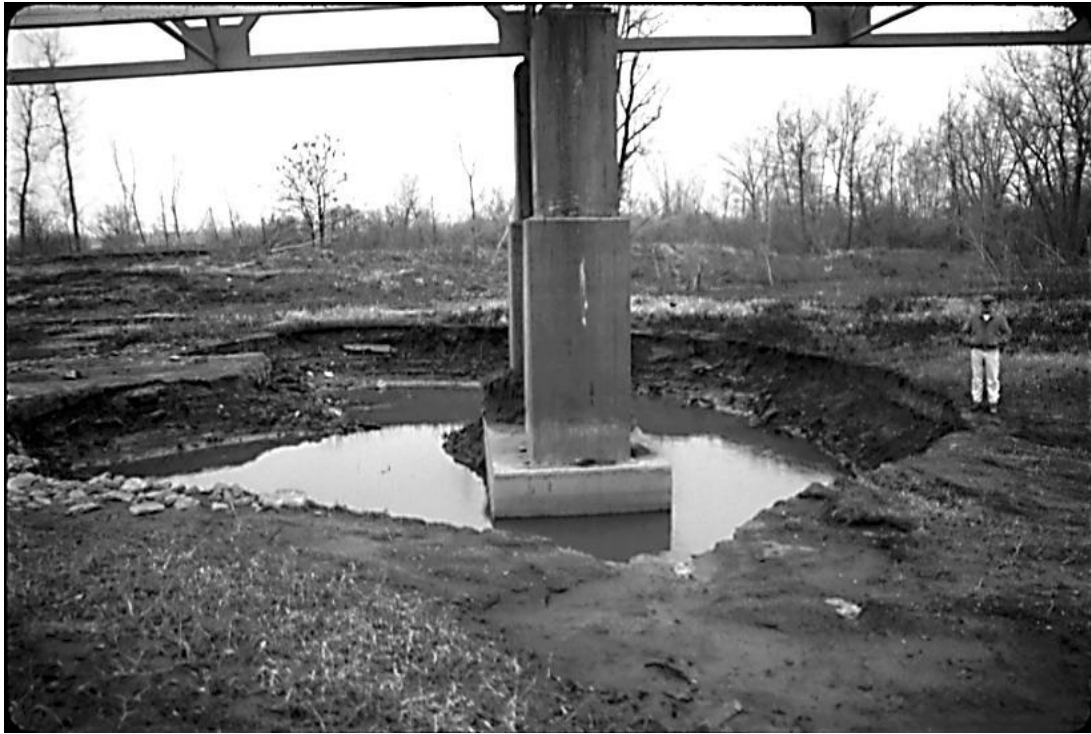
Figure 1-1 Local scour hole at a bridge pier after a flow event.
