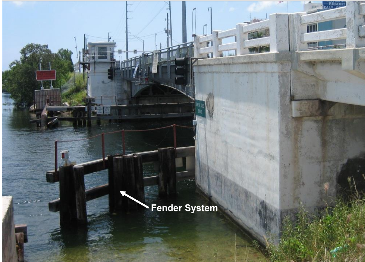
Figure 5.1-11: Fender System at the Old Jewfish Creek Bridge
