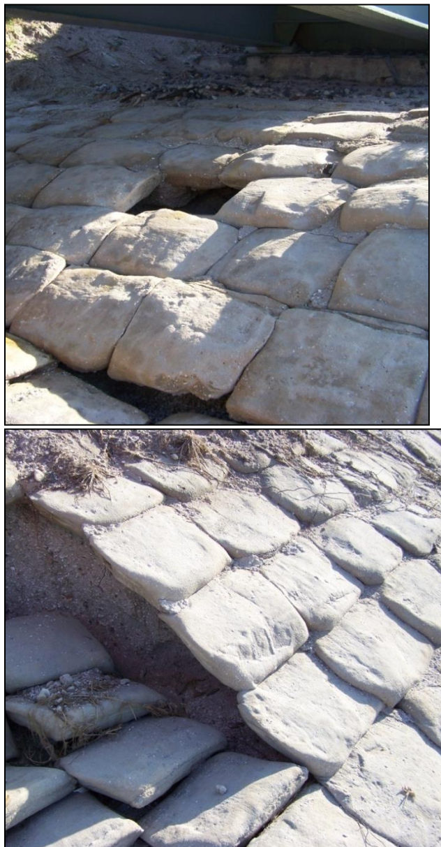
Figure 5.5-11: Damage to Sand-Cement Grouted Riprap Abutment Protection
