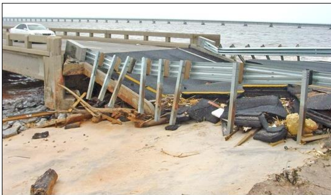
Figure 5.5-6: East Approach to the I-10 WB Bridge over Escambia Bay After Hurricane Ivan (2004)
