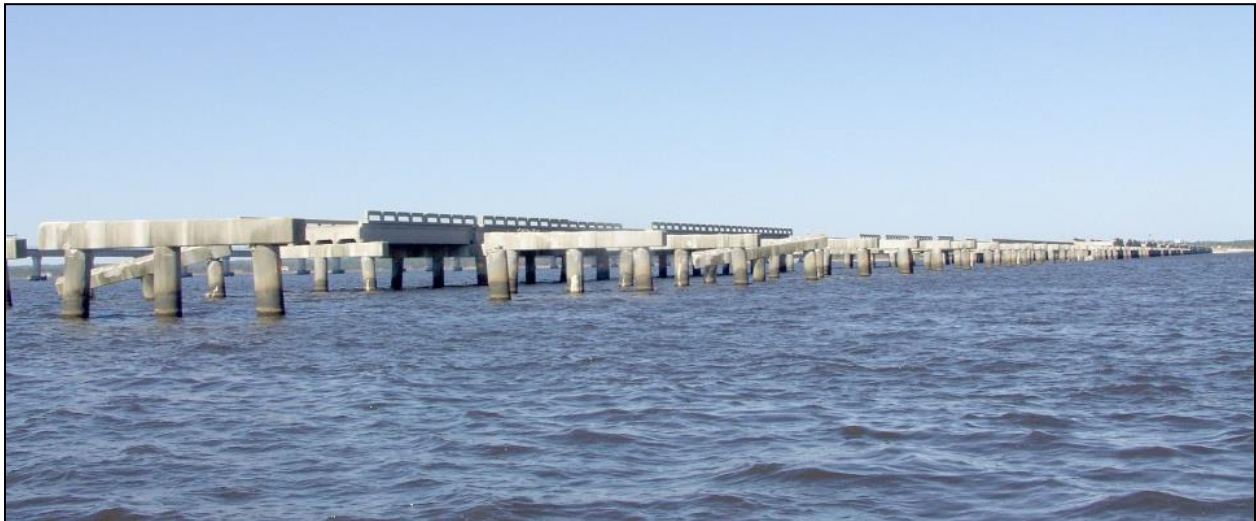
Figure 5.3-19: Damage to the I-10 Bridge over Escambia Bay during Hurricane Ivan (2004)
