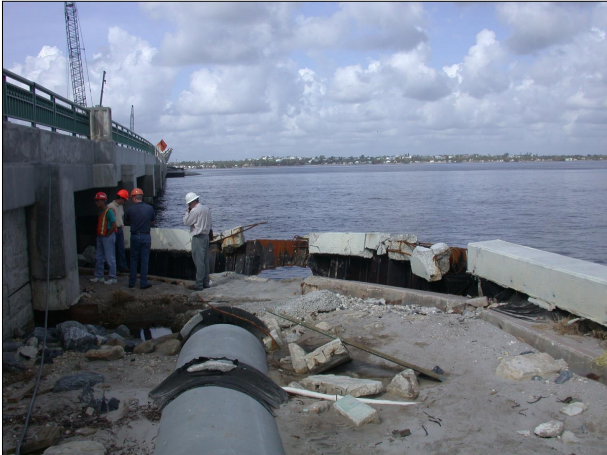
Figure 5.5-17: Seawall Failure Following Hurricane Frances (2004)
