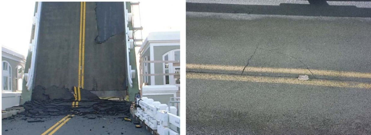
Examples of wearing surface failures
