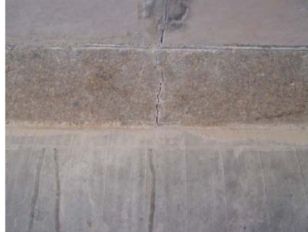
Crack in Haunch
