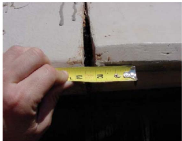
Misalignment of Deck-to-Deck Joint
