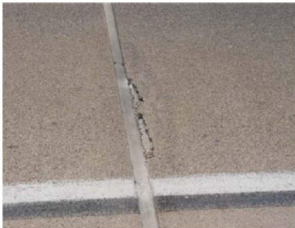
Debonding at Joint and below Wear
