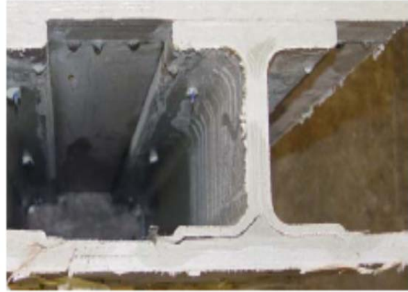
FRP Delamination (ZellComp)
