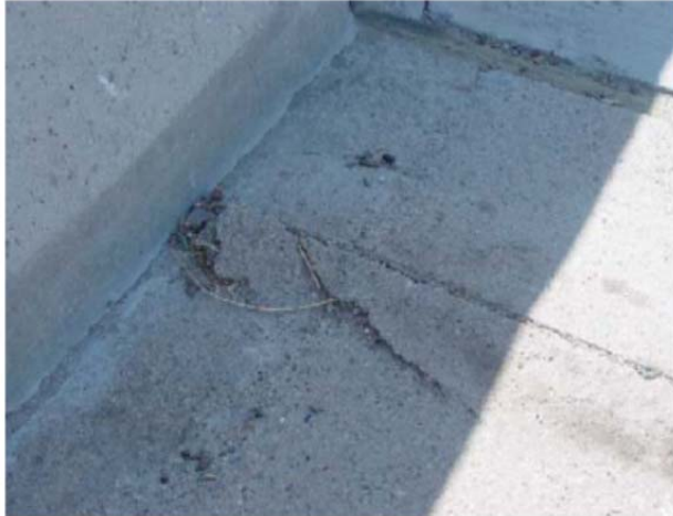
Buckling of Wearing Surface
