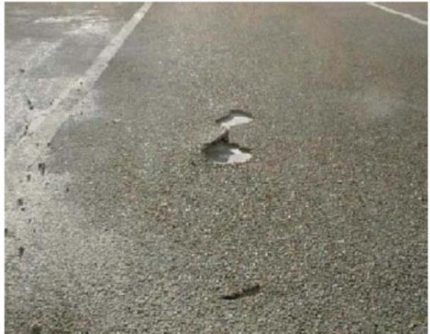
Wearing Surface Debonding
