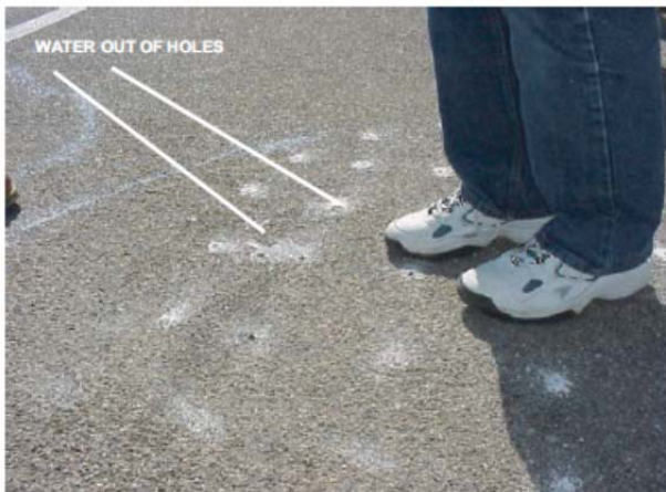
Water found within core of deck after drilling
