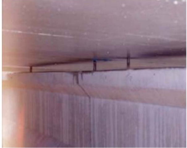
FRP Deck and Connection Studs Separation
