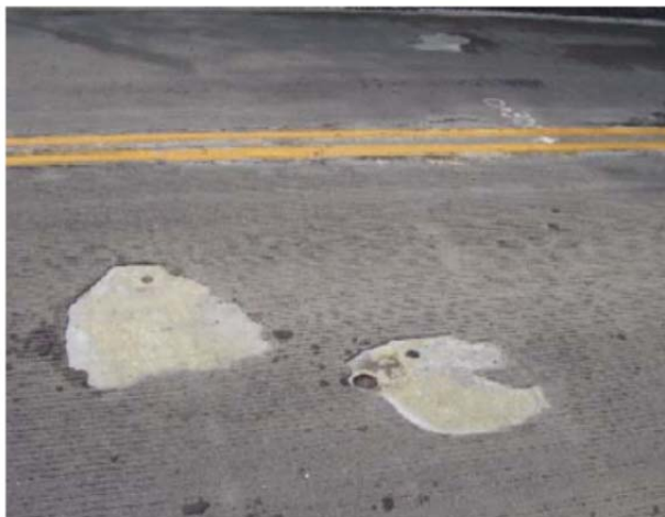
Delamination of Wearing Surface
