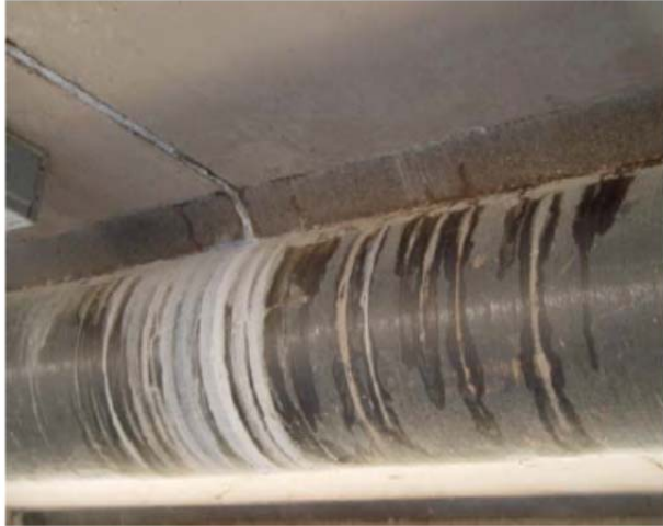
Leakage through Deck-to-Deck Joint
