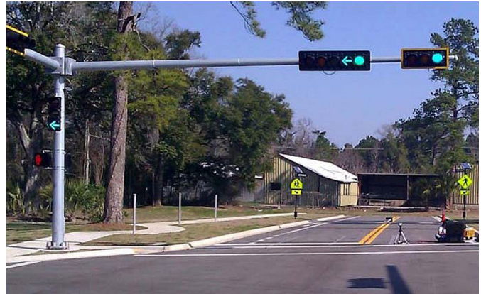
These test track signals display safety features, including redundancy and black housings with orange surrounds. Researchers investigated the effectiveness of the pedestal signal, visible at the left of the image.
