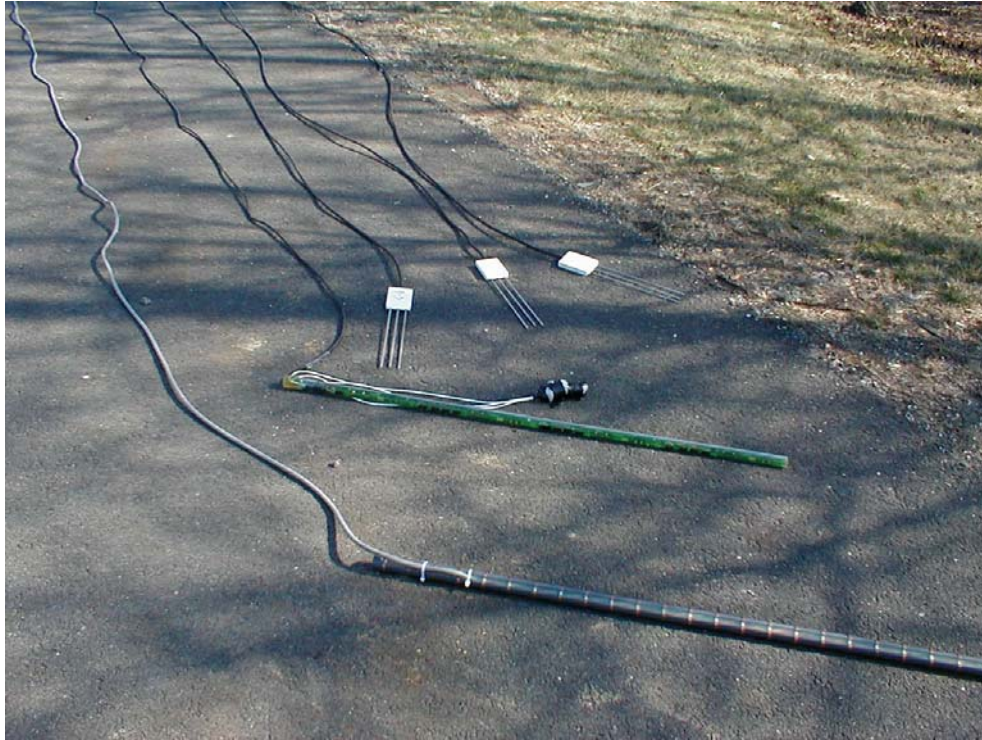
Figure 3- TDR (top), temperature (middle), and resistivity (bottom) probes to be installed in test section 3.
