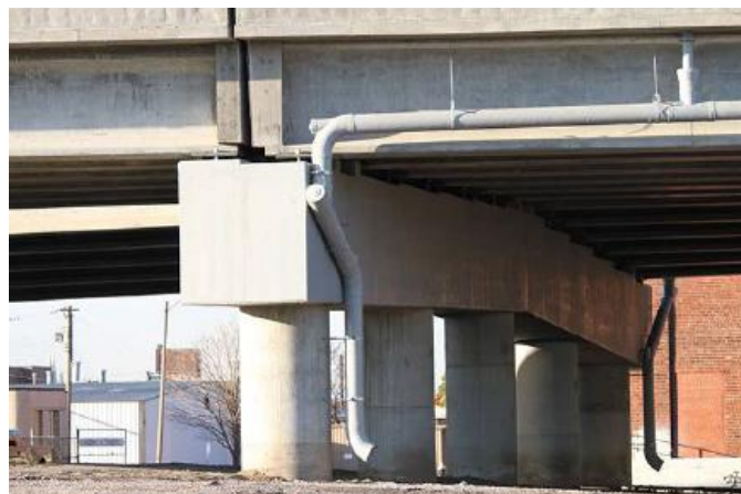
Figure 10.27 Closed Bridge Drainage System with Steeper Pipe Slopes, Long Radius Bends and Cleanouts (Courtesy of FRPbridgedrainpipe.com)
