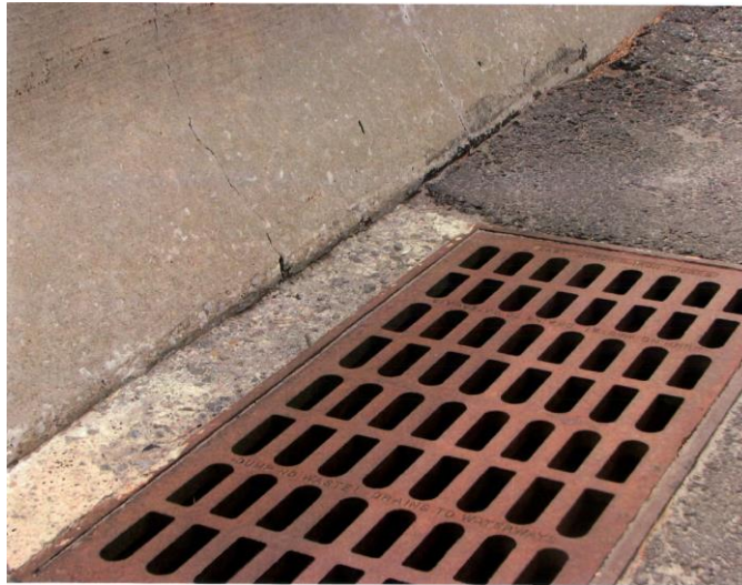
Figure 10.24 Bridge Inlet Grate Retrofit (Filter Grate) (Courtesy of the New Jersey Turnpike Authority)
