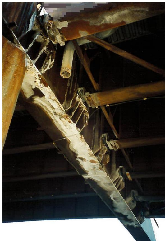
Figure 10.20 PVC Drain Extension Retrofit Beneath Deck (Courtesy of the New Jersey Turnpike Authority)
