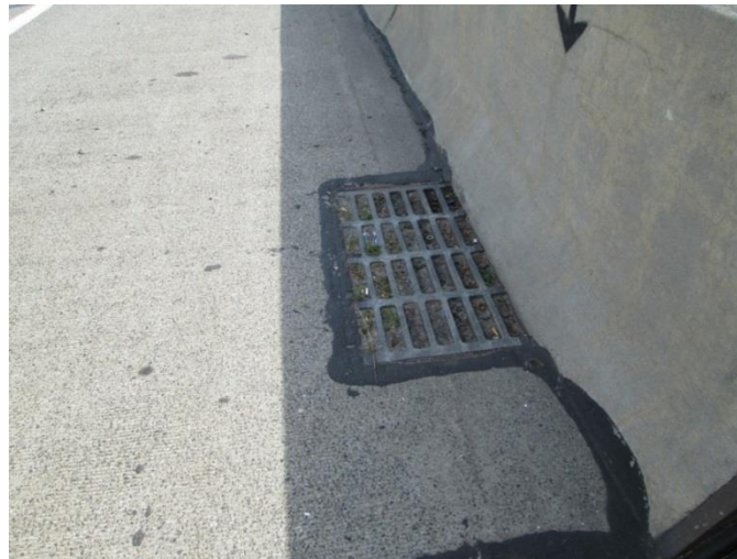
Figure 10.22 Bridge Inlet Grate Which Permits Clogging of Inlet (Courtesy of the New Jersey Turnpike Authority)
