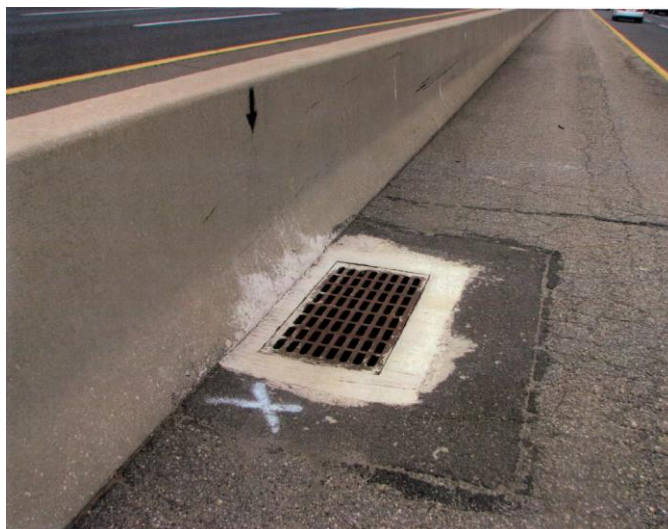
Figure 10.25 Bridge Approach Inlet Grate Retrofit (Filter Grate) (Courtesy of the New Jersey Turnpike Authority)
